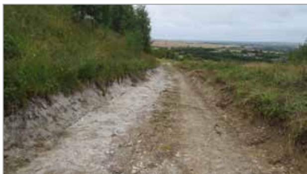
The alternative sunken way used for the work just after the cables were laid underground. Photo by Graham Bellamy
